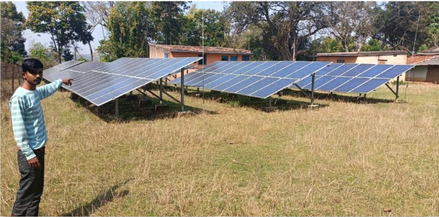
Mini Grid Operator showing the solar panel set-up, Simdega, Jharkhand
