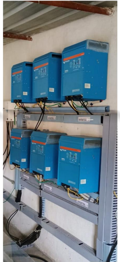
Battery Backup of a Solar Mini Grid, Gumla, Jharkhand
