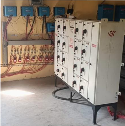
Set-up of a Solar Mini Grid, Simdega, Jharkhand
